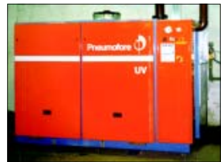
Fig 1 - UV 30 vacuum pump installed at the Owens-Illinois plant in Nove Sedlo, Czech Republic, May 1999
